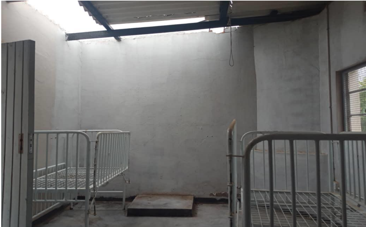
Fig 3. The Children's Nursery was damaged by strong winds during Cyclone IDA1 phase
