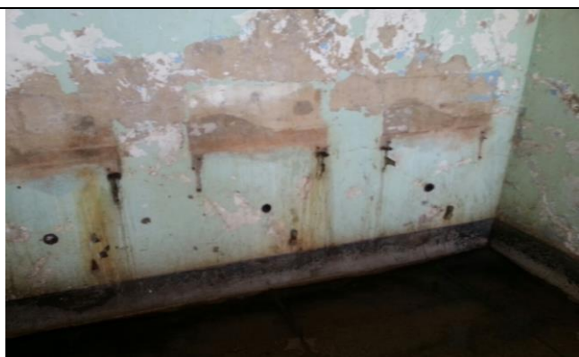
The photo above shows the interior of a bathroom, where sinks have been destroyed by the patients
